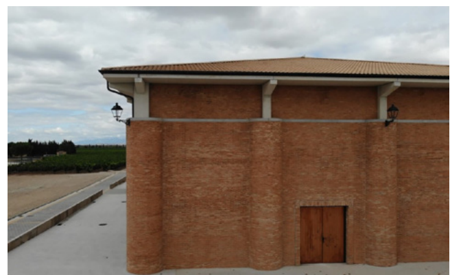
Figure 6. Image of the building envelope taken by the drone during the first inspection flight.
