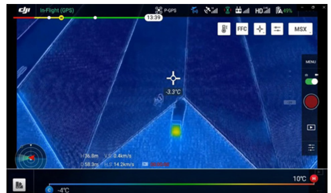
Figure 9. Temperature differences detected by the thermal camera: Flue in the roof.
