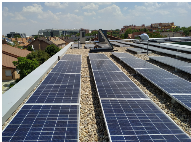
Figure 3. Photovoltaic solar panels on the rooftop.
