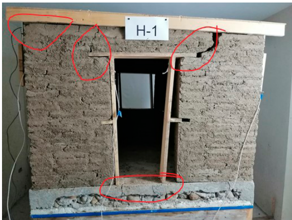
a. Large cracks around the door opening, front view
