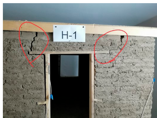
Figure 14. Cracks around the door opening, front view
