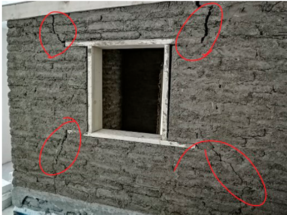
Figure 15. Cracks around the window opening, back side view
